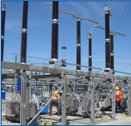
High-voltage switchgear during factory acceptance testing. Photo: US ITER
