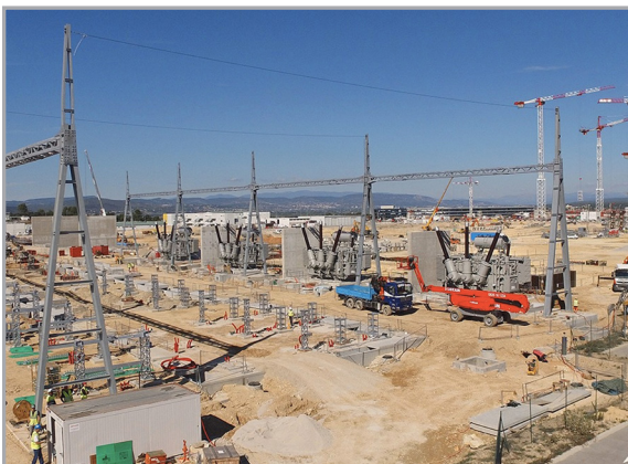
A wide view of the installed high-voltage transformers and the electrical gantry train. Photo: ITER Organization
