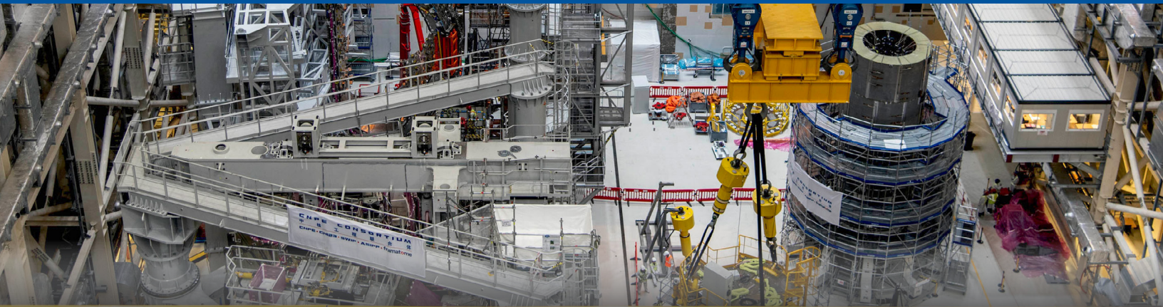
Numerous activities are underway in the ITER Assembly Hall, including vacuum vessel sector (left) and central solenoid assembly (right). Photo: ITER Organization
