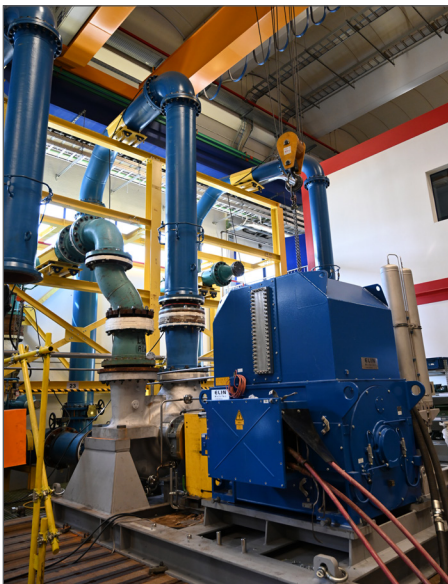
Assembly is complete for this primary pump of the vacuum vessel heat transfer system. Photo: US ITER
