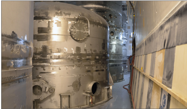
Drain tanks produced by Joseph Oat Corporation in Camden, NJ, were the first U.S. components installed in the tokamak complex. Photo: US ITER
