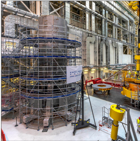
The fourth module installed on the central solenoid stack. Photo: ITER Organization
